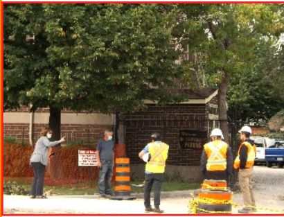
AREA property owner gives City crew an earful. (above) Trees to be removed at right.
