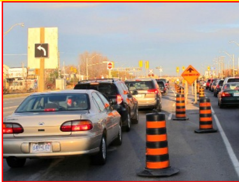
EXPECT SOME DELAYS as a watermain replacement project clogs up Lake Shore Blvd. W., in Long Branch.
