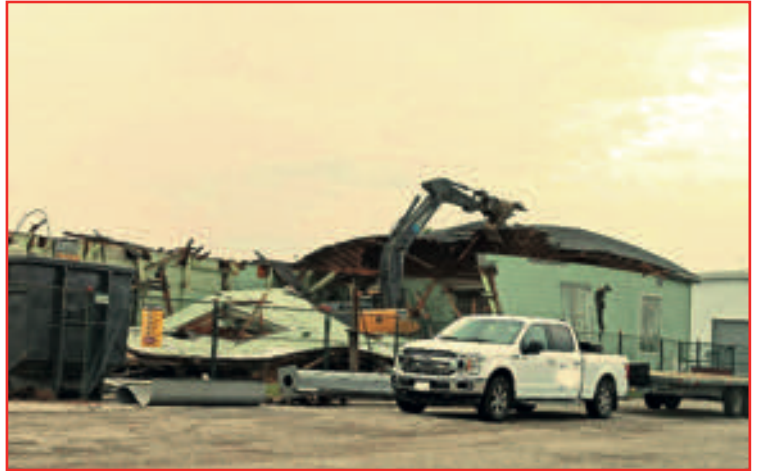
THE LAST OF THE AIR HANGARS at CFB Borden are being demolished as time marches on and with many memories gone. Many South Etobicoke flyers trained here. Photo by Garfield Ingram.
