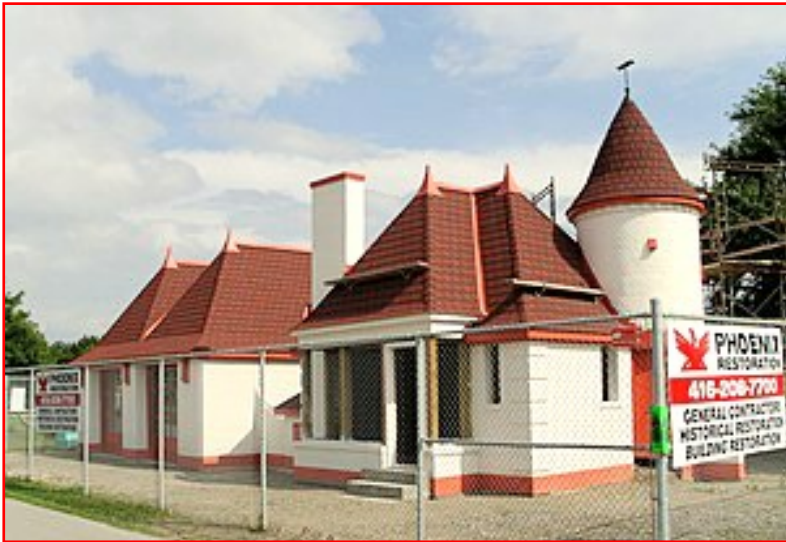
THE HISTORIC JOY OIL station on Lake Shore Blvd. W., has been renovated and sitting idle for many years.
