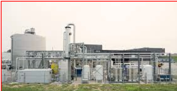
SECTION OF THE processing system used to convert some of Toronto's garbage into heating gas.
