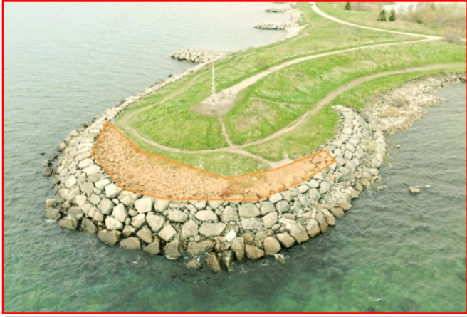
ANTI-FLOODING WORK to some shoreline at Colonel Samuel Smith Park is expected to take a year or more and cause some path closures. Courtesy photo.
