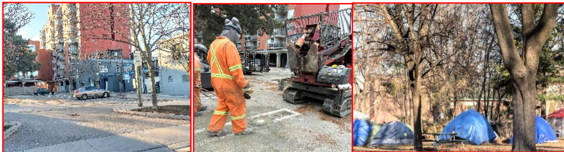
CITY CREWS (centre) BEGIN WORK ON an 80-bed municipal shelter for the homeless (right) being constructed on Third Street (left). Some residents claim ‘enough is enough,’ and call for community consultations..
