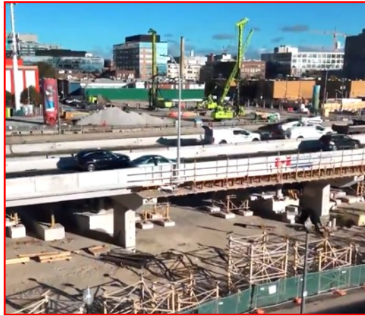
CONSTRUCTION underway at a highway bridge. Five bridges will have to be restored in big job.
