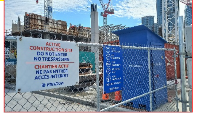
BUSY CONSTRUCTION site at the Six Points Interchange as crews build a new Etobicoke Civic Centre.
