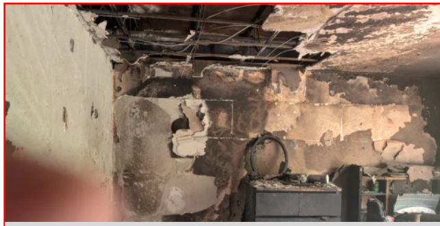
INTERIOR DAMAGE caused from the lithium battery fire (above) Firefighters battle a similar battery blaze (below).
